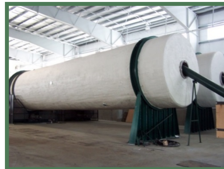
Figure 9: Rotating Drum System
