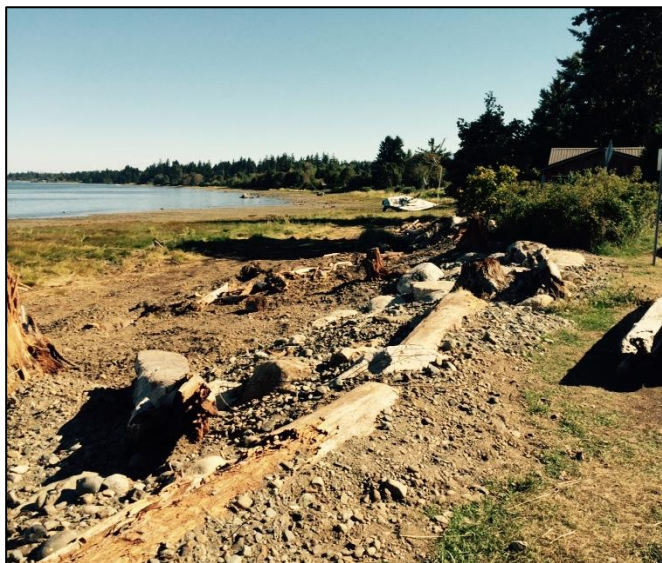
Figure 4. Example of installed Large Woody Debris revetment along another shoreline in the Comox Valley.
